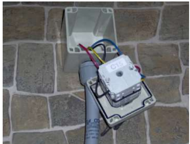
4 x 14 gauge wires used for key switch
